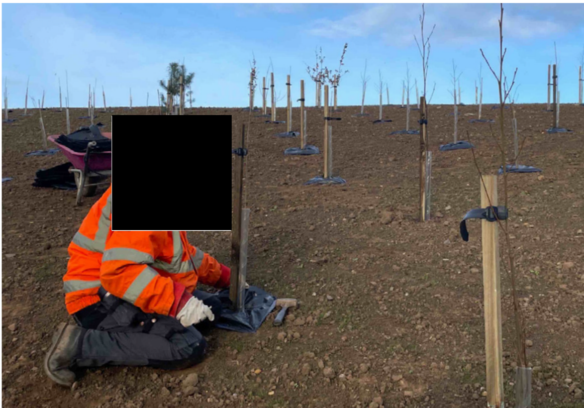
Example of revegetation underway at converter station site (Sofia and Dogger Bank C)
